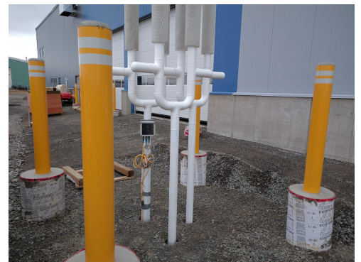
D505 Logger mounted on a thermosyphon with Digital Temperature Cables connected.
