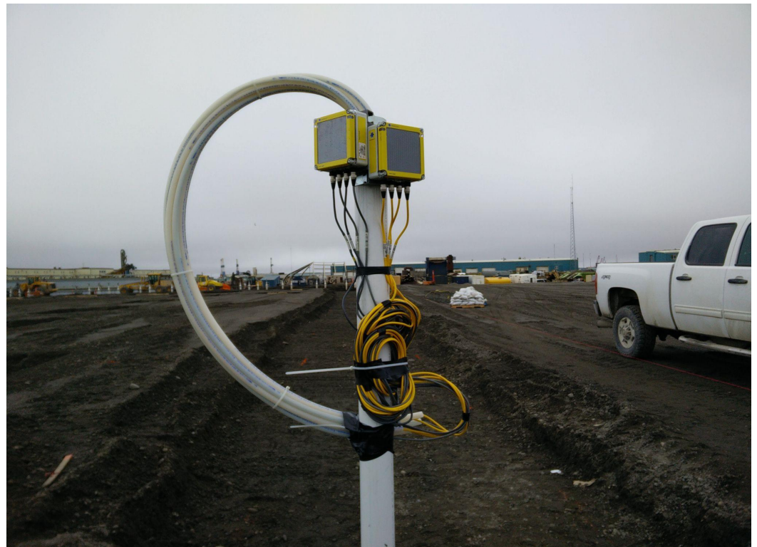
Eight DTCs connected to mounted D405 satellite data loggers for seamless monitoring.
