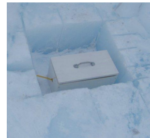
Custom-built boxes for beadedstream's temperature monitoring gear at Wilkins Runway.
