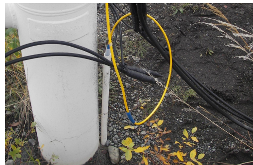
beadedstream's Digital Temperature Cables installed in the ground with a PVC conduit.
