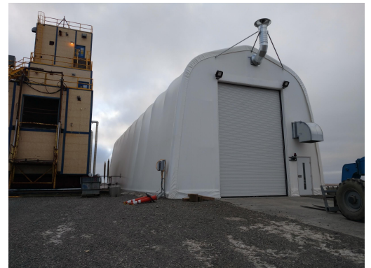
Exterior of the truck off-loading tent, note the mounted panel box with Digital Temperature Cable outside (left side of building).
