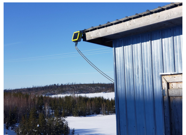
D505 data logger mounted on the sump building roof, collecting data from 2 digital temperature cables.
