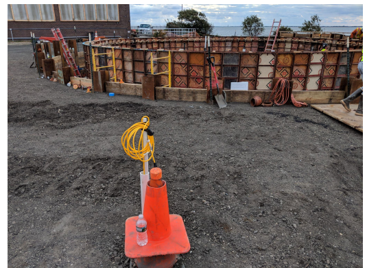
A Digital Temperature Cable in the foreground with the launch shaft in the background.
