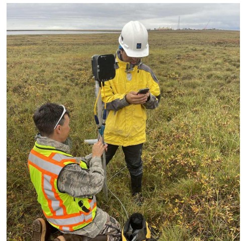
Tundra temperature sensors are installed in the fall before the ice road construction season starts.
